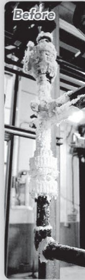
Leaking sodium hypochlorite in a welded PVC system
